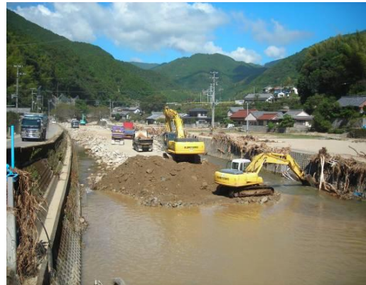
Figure 18: Emergency removal of earth from waterways
