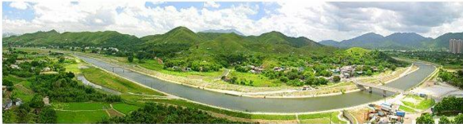
Completed river training works at Ng Tung River near Tin Ping Shan, Sheung Shui
