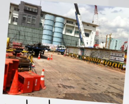
steel plate access
