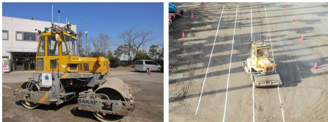
Figure 14 – Verification Tests of un-manned Machinery
