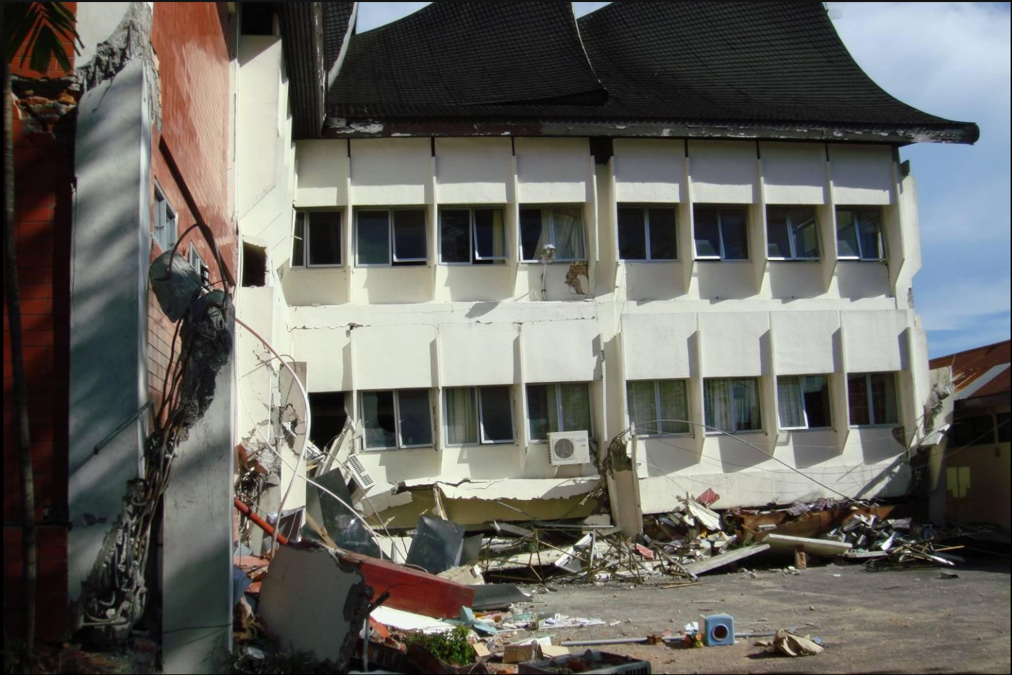
Soft story collapse of a Government building (Courtesy: Teddy Boen)
